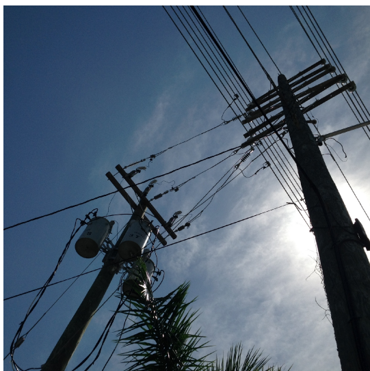
Photo: 13 kilovolt (kV) distribution and 69 kV transmission lines on Grand Cayman.
