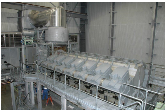
Photo: 16 MW diesel generating set at CUC's North Sound Plant.
