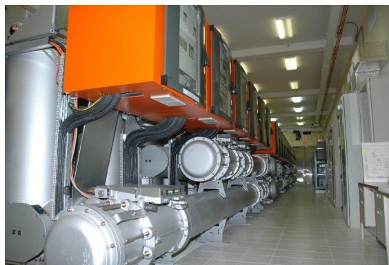
Photo: Switchgear inside a CUC substation on Grand Cayman.
