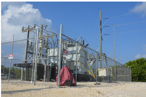
Photo: Mobile substation in Prospect on Grand Cayman.
