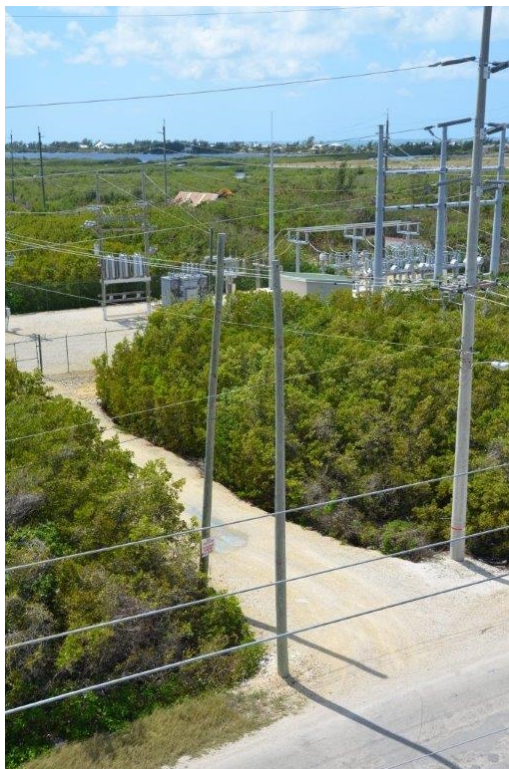
Photo: Aerial view of Rum Point substation on Grand Cayman.
