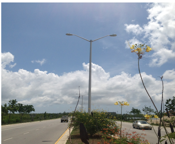
Photo: High pressure sodium street lights on Grand Cayman.
