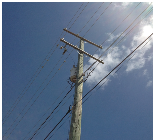
Photo: Distribution pole carrying electricity and communications lines.
